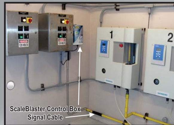
ScaleBlaster is installed on the City of Stuart, Florida Reclamation Facility and removed all limescale formation from the chlorine lines & electronic valves. This freed up an employee from having to spend one day a week cleaning them out.
