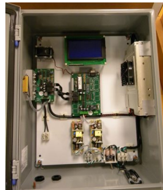
Control unit with door opened showing electronics inside
