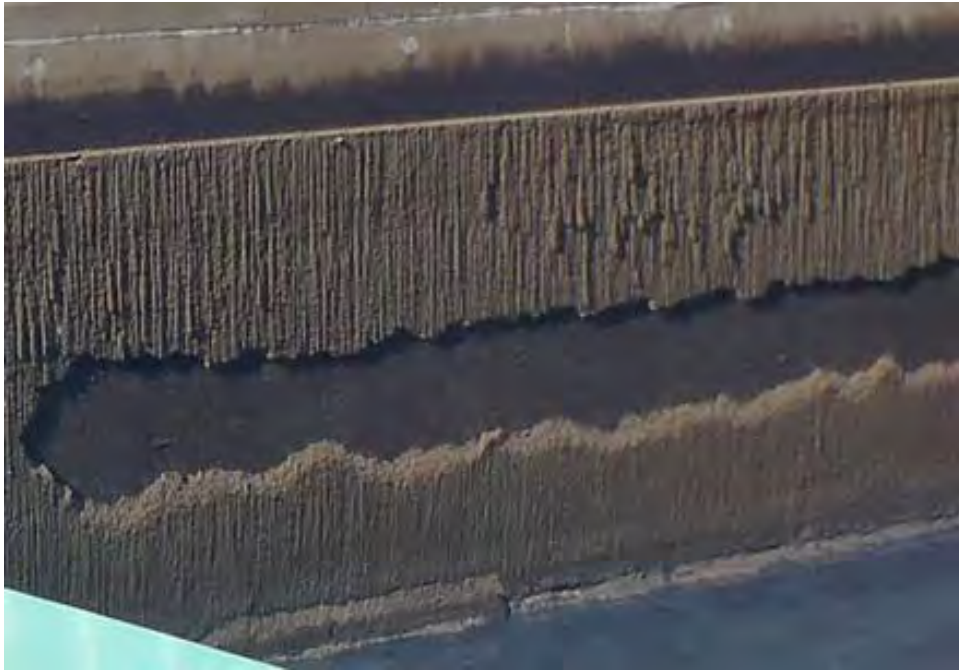
Photo 12: Clarifier Wall taken May 2, 2012 (Clarifier in service for 16 months)
