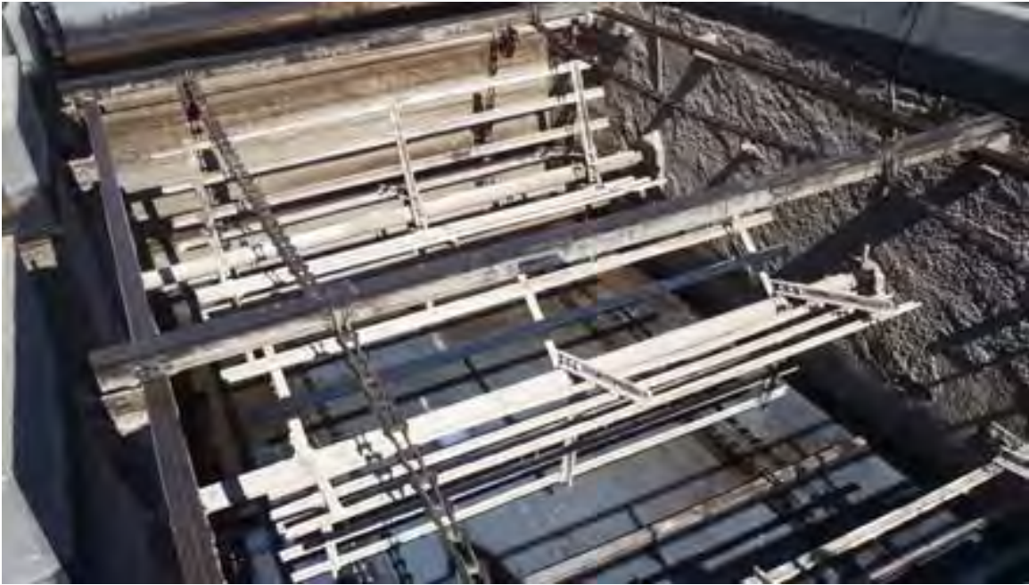
Photo 16: Flocculation Chamber taken April 28, 2015
