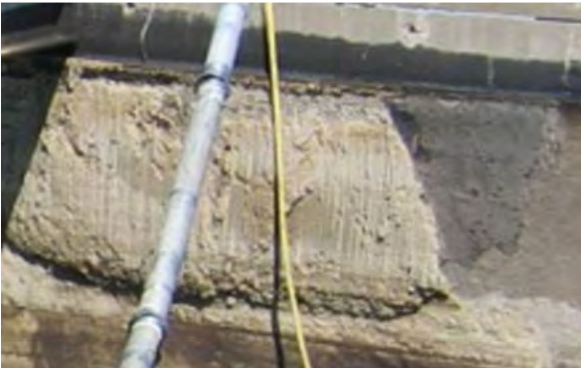
Photo 11: Clarifier Wall taken April 2, 2007 (Clarifier in service for 6 months. Part of wall already scraped)
