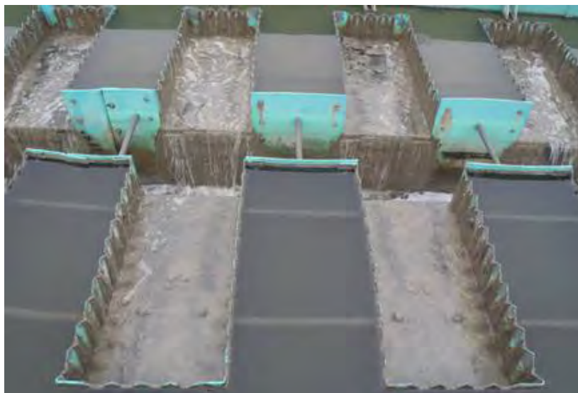
Photo 6: Clarifier Weirs taken December 22, 2011 (1 month of no cleaning prior to ScaleBlaster)
