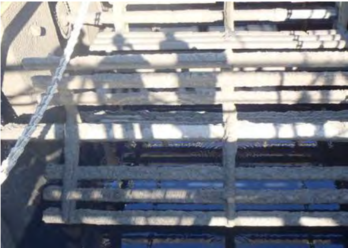
Photo 15: Flocculation Chamber taken May 2, 2012 (close up)
