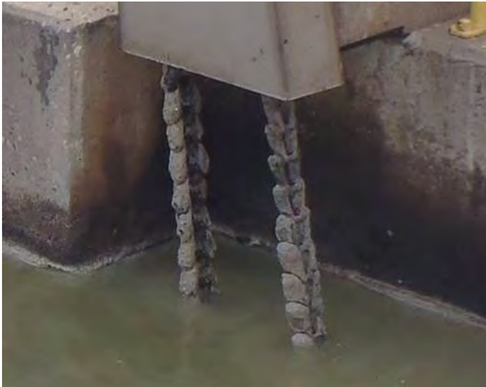
Photo 9: Flocculation Chamber Chains taken January 30, 2012
