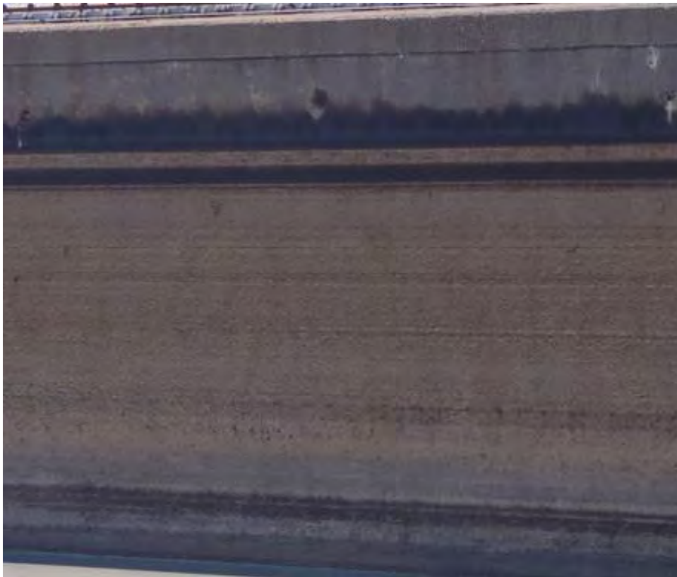
Photo 13: Clarifier Wall taken April 28, 2015 (Clarifier in service for 6 months)
