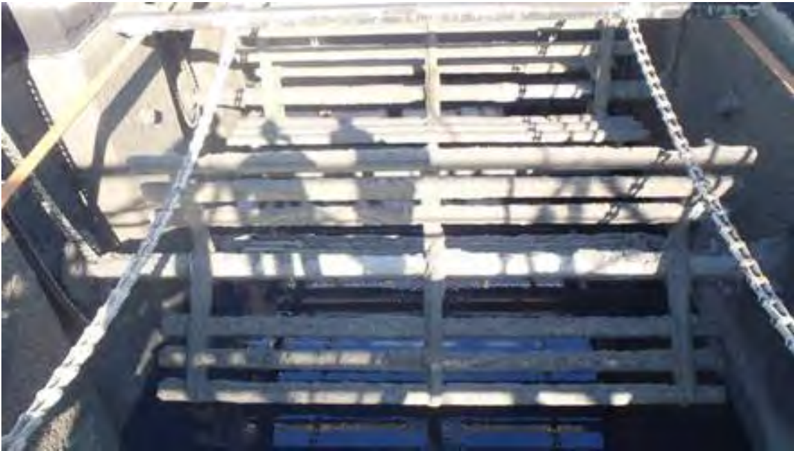
Photo 14: Flocculation Chamber taken May 2, 2012
