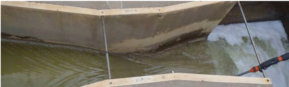
Photo 1: Effluent Flume taken January 31, 2012
