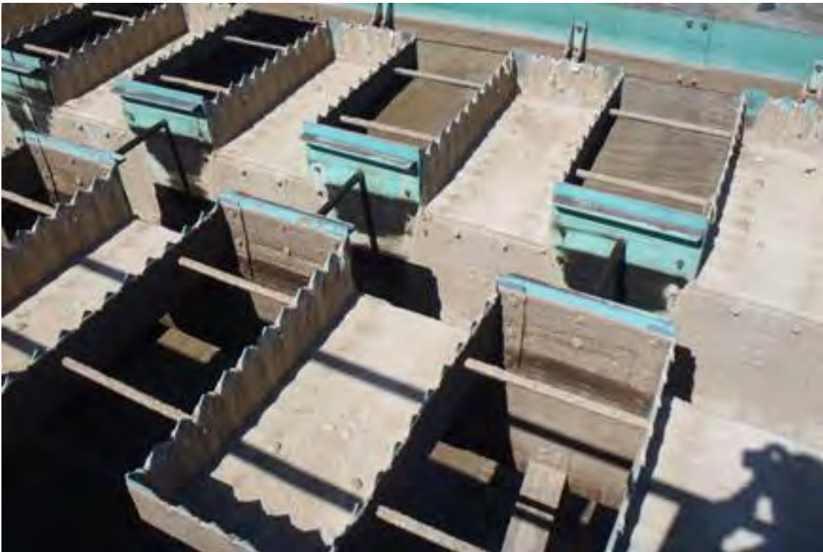
Photo 8: Clarifier Weirs taken April 28, 2015 (Clarifier taken out of service April 22, 2015. No cleaning since November 5, 2014 when clarifier was put in service)
