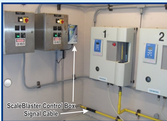
The City of Stuart (FL) Water Reclamation Facility uses ScaleBlaster to clean out the chlorine lines & electronic valves which results in huge labor savings & downtime.
