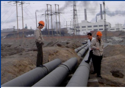
Shizuishan Power Plant - Yinchuan, China
