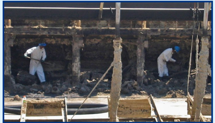
American Bottoms Wastewater Treatment Facility in Sauget, Illinois has dramatically decreased the time needed to clean their clarifiers
