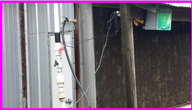
ScaleBlaster installed on a cool pad at a Georgia poultry farm
